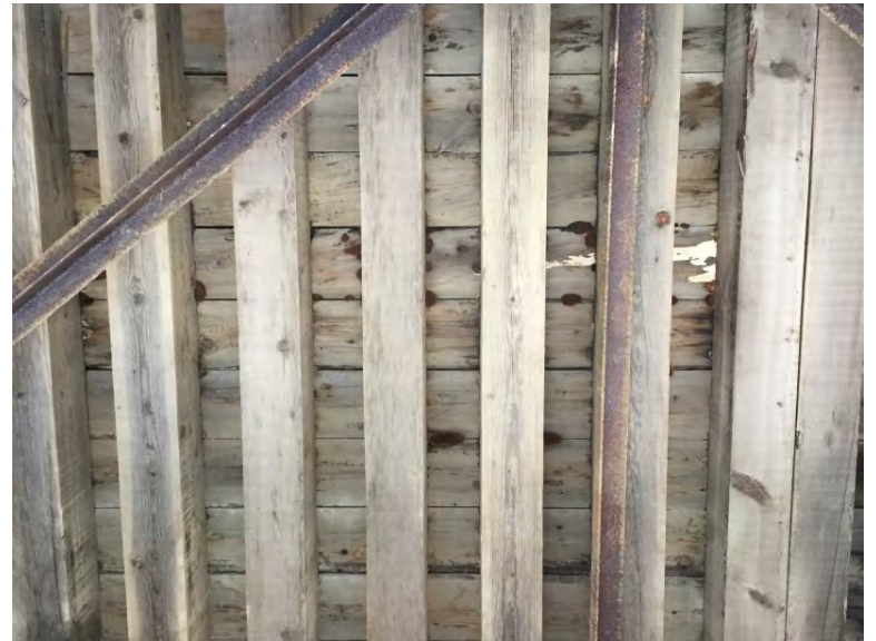
Subdeck condition at midspan
