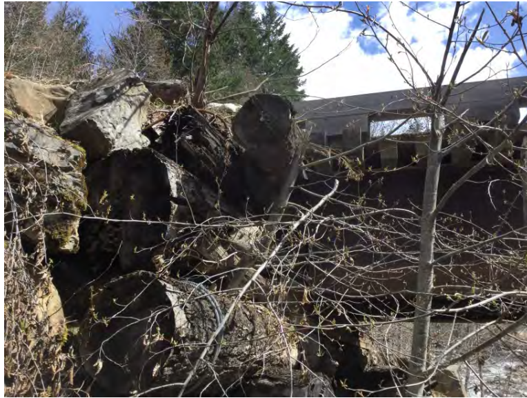
Top log of ballast wall at right bank is failing
